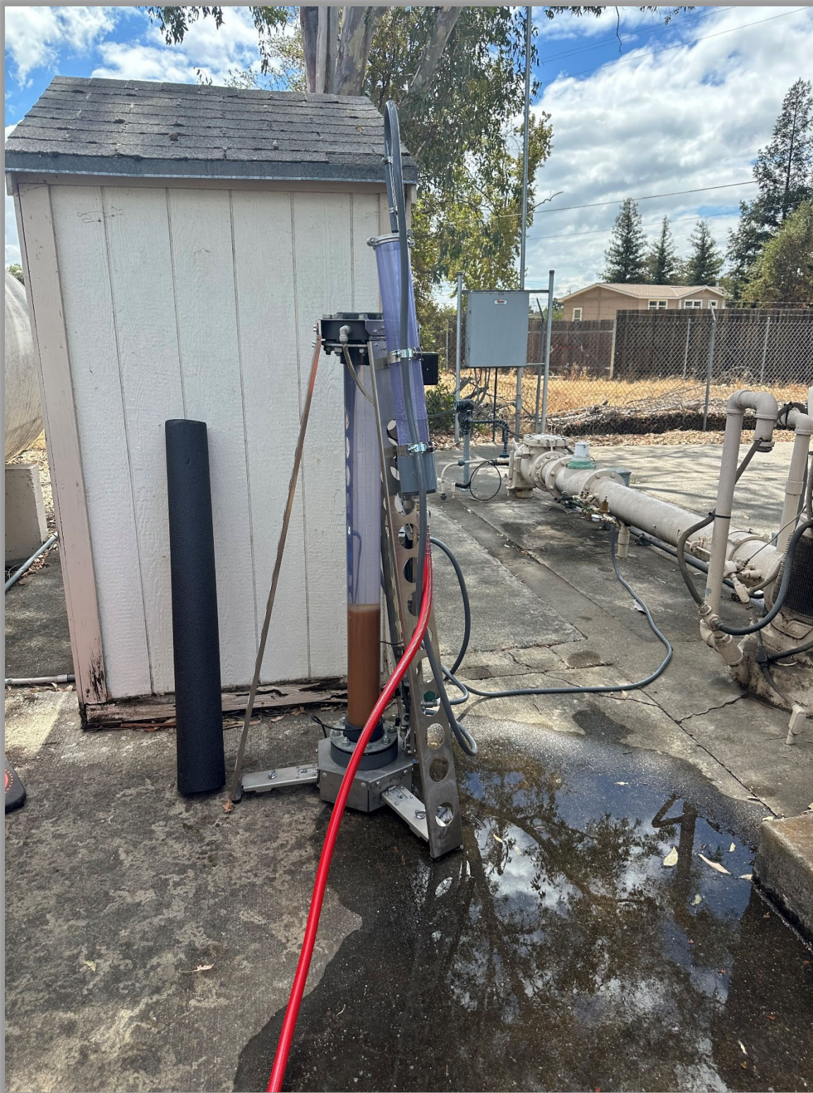
Cr6 SBA-IX Treatment Pilot System Installed and Operational at Well 10
