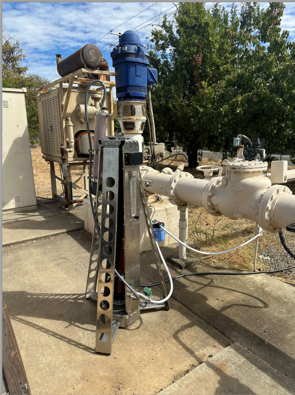
Cr6 SBA-IX Treatment Pilot System Installed and Operational at Well 2A
